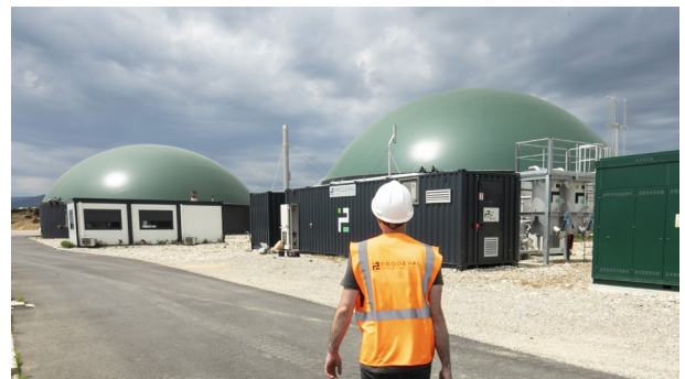
A world first in the Biogas sector! Photo Credit: PRODEVAL
